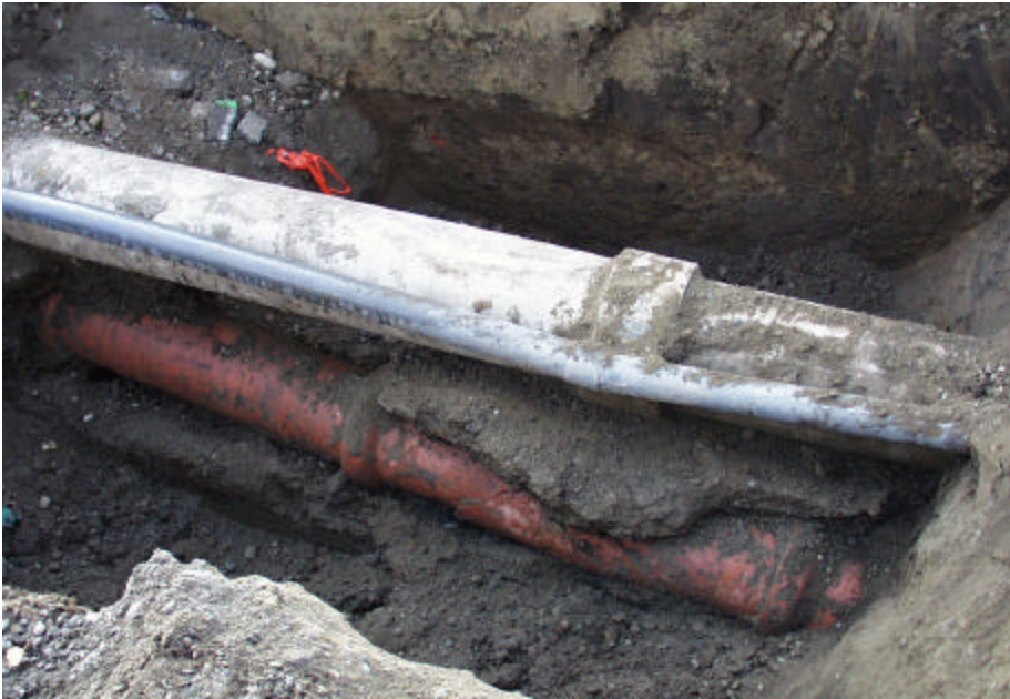
Figure 3. On Marine Drive, broken 12" diameter clay sewer pipe below water pipe and electrical conduit. (September 2001) Photo by Jon Walter
