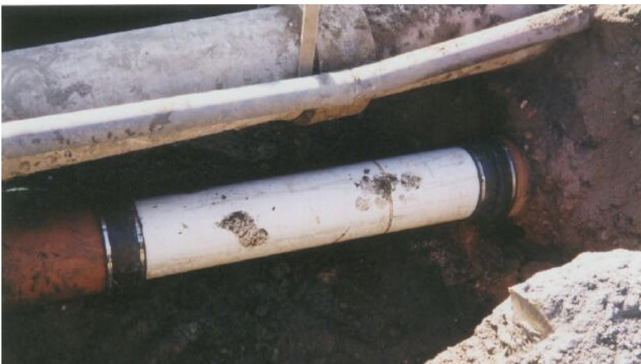
Figure 4. On Marine Drive, 12" sewer pipe repairs completed by Public Works (September 2001) Photo by Jon Walter
